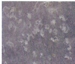
Damage by Salt
