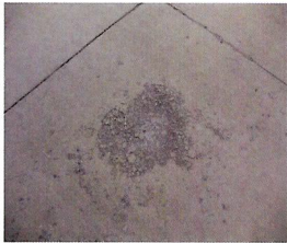
Damage by Deicer
